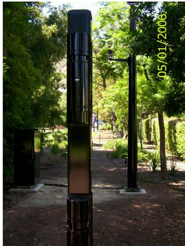
Perimeter PE Beams with Camera and Enclosure in background
